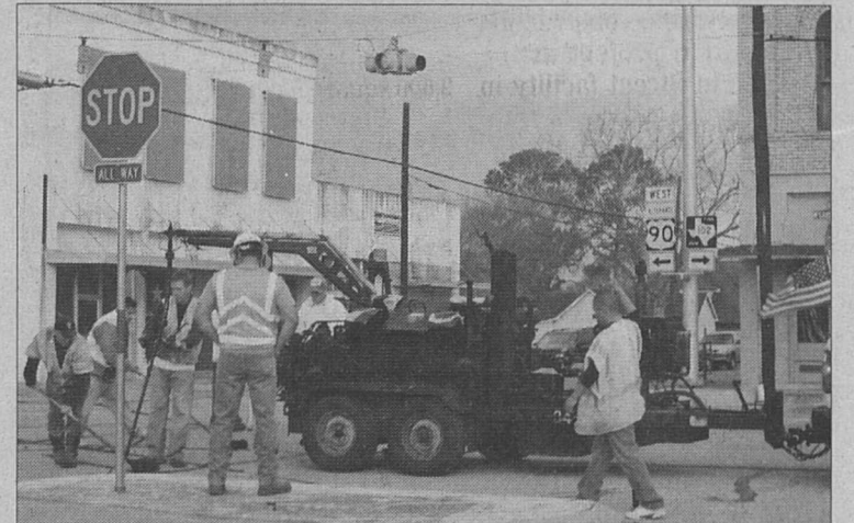
Contractors were downtown on Monday, Feb. 16 in Eagle Lake performing crack sealing on the roads. Texas Tree and Landscape Ltd. of China Springs was handling the work for the Texas Department of Transportation.
